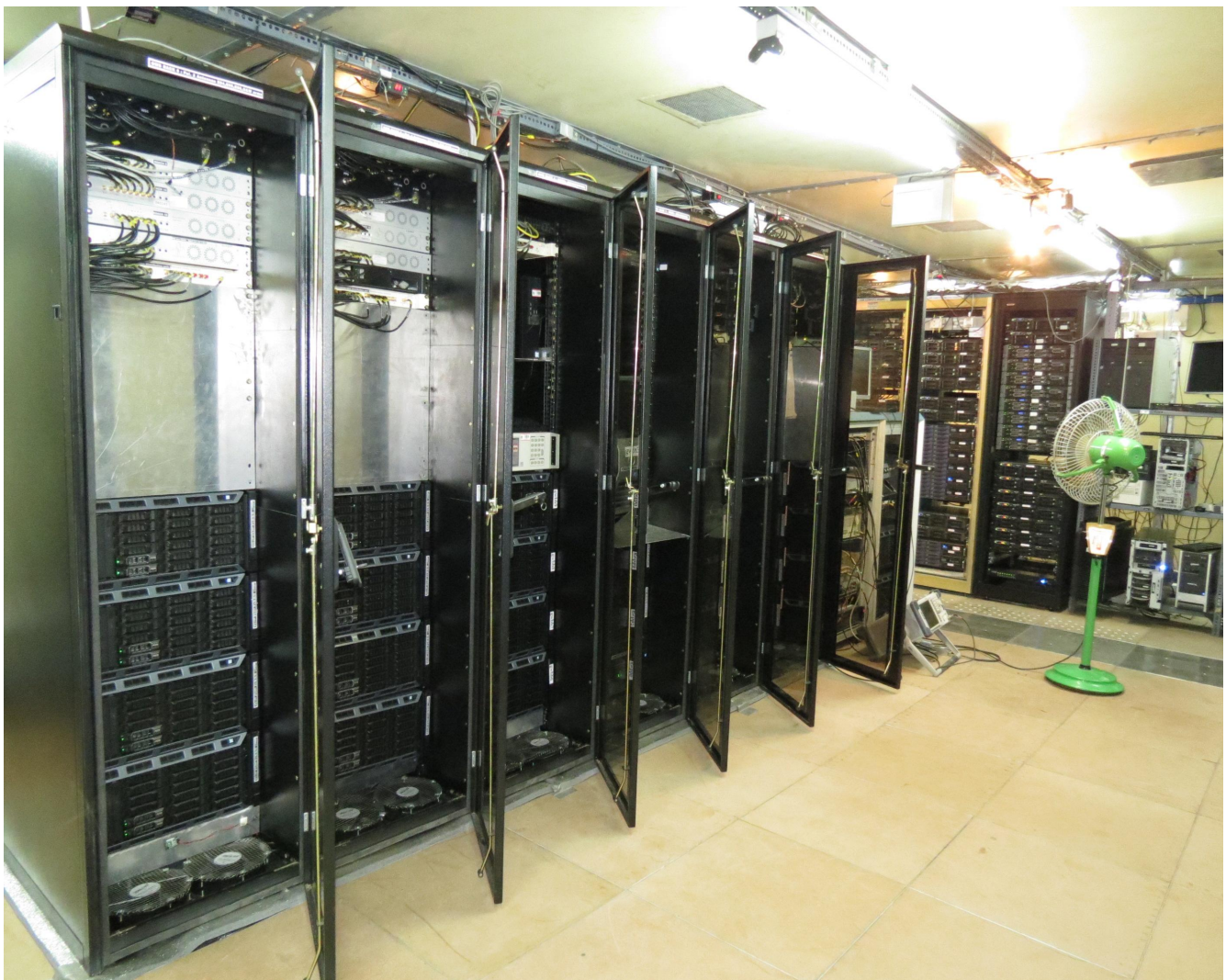
Image 1 : 30 Antenna GWB system integrated in 6 racks..
