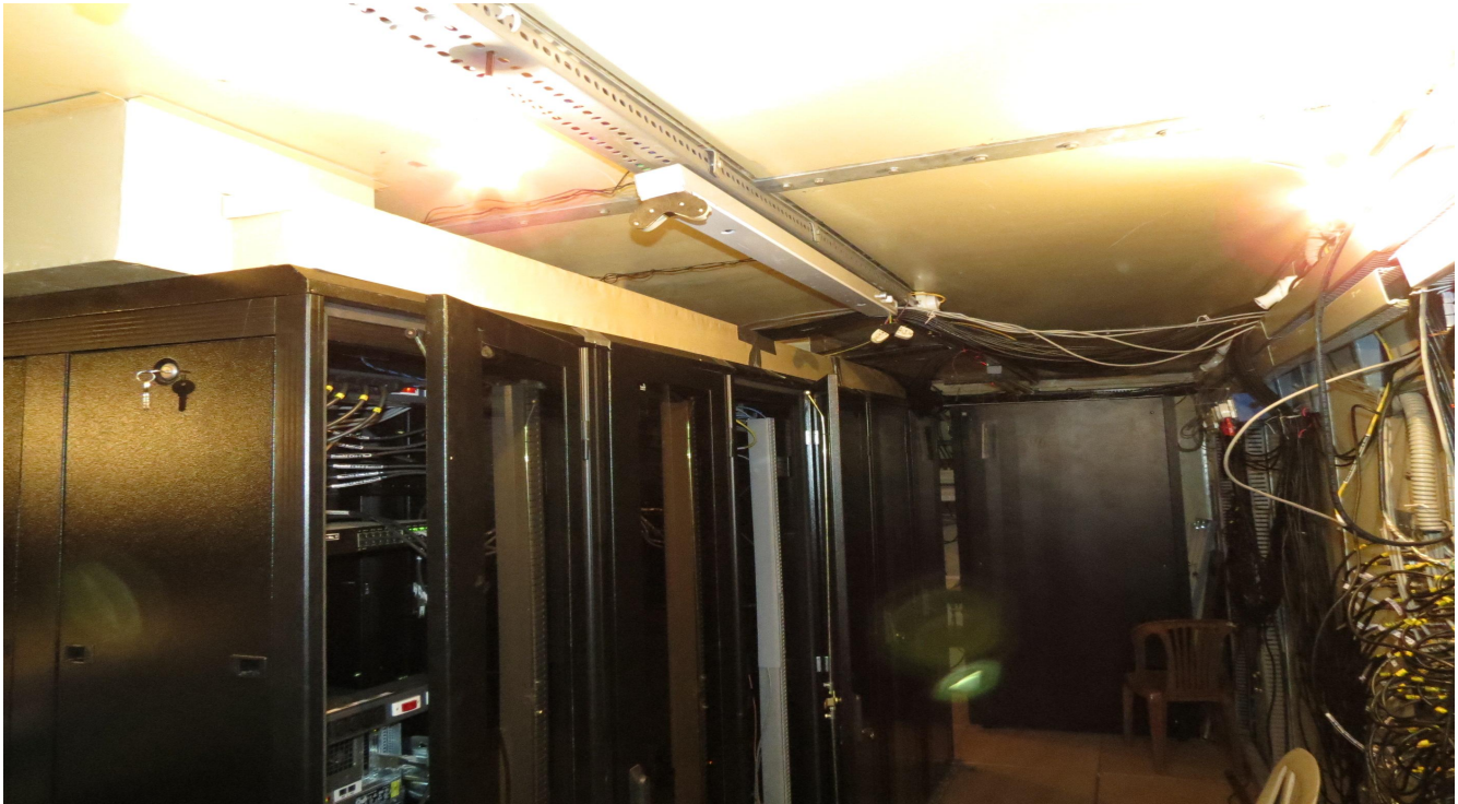
Image 2 : Back view of the 30 Antenna GWB system with outlet hot air duct above the racks.
